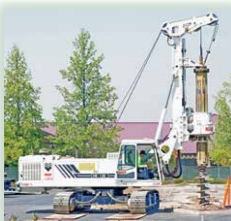
Solar Works drilling holes for footings for placement of the Solar Panels
