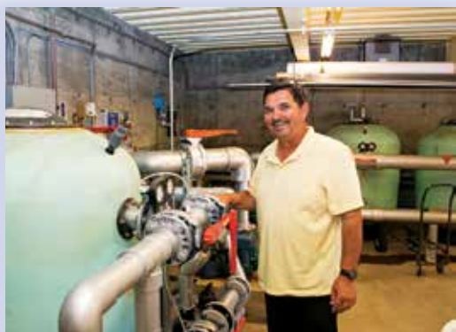
Dave in the Pump Room
